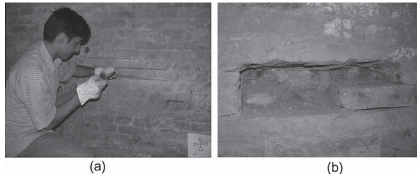
Fig. 6. Removal of the bricks from the walls. (a) Remove-brick-operation. (b) Hole in the wall after the removal of a brick.
