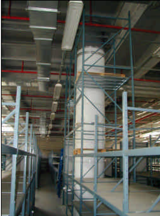
fig. 10: Duct unit (D = 90 cm, L ≈ 13 m).
